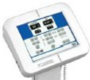
Touch screen panel outside room at the work station.
